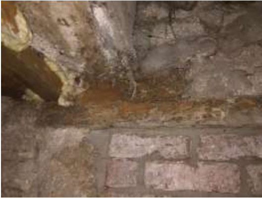
Photo 65 - Room G5 – Rot to lintel over infilled opening into Room G1.
