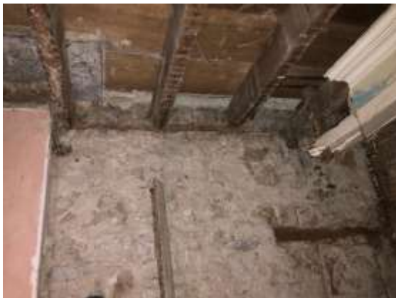
Photo 38 - Room G1 – Rotten ends to floor joists and bearing timber.
