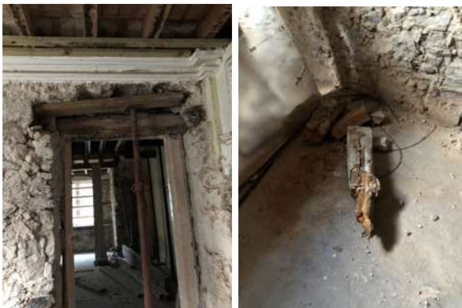
Photos 59 & 60 - Room G7 – Failure of timber lintel to doorway through to Room G3 due to rot.
