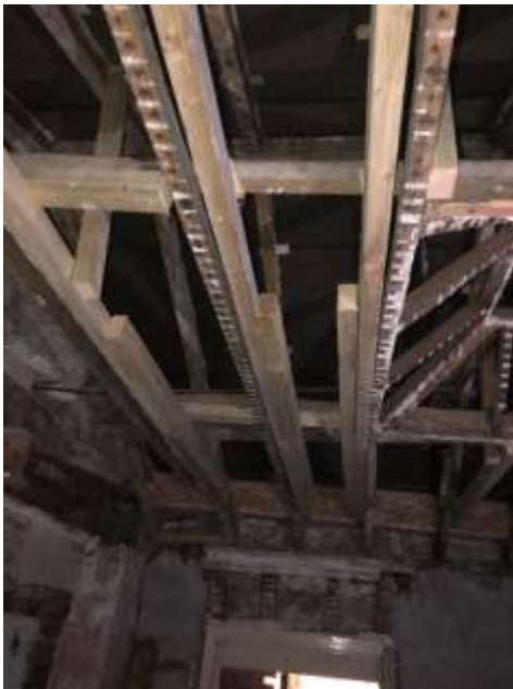
Photo 58 - Room G3 - Splicing, bracing and replacement of rotten roof and ceiling timbers.
