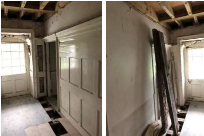
Photos 49 & 50 – Warping to wall paneling due to presence of dry rot, missing paneling to opposite wall.
