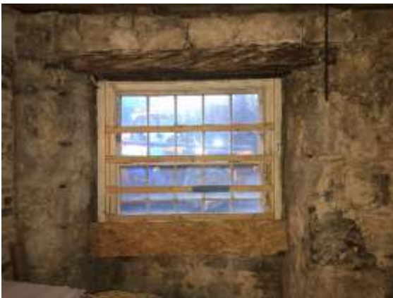
Photo 72 - Room G8 – Rot to lintels above window W15.
