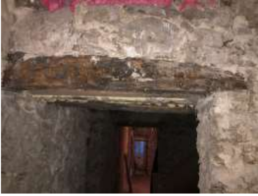
Photo 68 - Room G7 – Rot to lintel over opening leading to Room G6.
