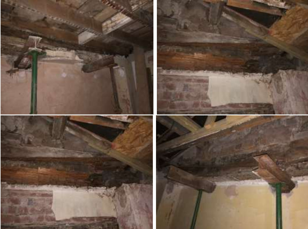
Photos 54 to 57 - Room G3 – Rot to supporting beam between this room and G2 with corrosion to previous diagonal steel bracing bars.
