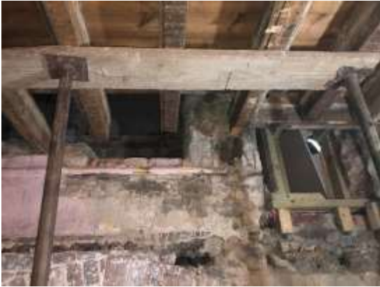
Photo 71 - Room G8 – Rot to ends of floor joists cut out and temporary supported until repair can be carried out.
