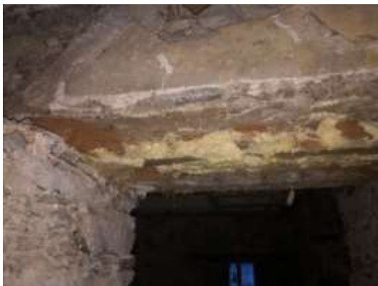
Photo 64 - Room G5 -Rot to lintel over opening leading to Room G6, previous use of expanding foam evident, purpose unknown.
