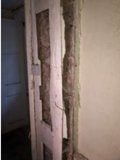
Photo 40 - Room G1 – Dry rot to right hand door frame in G1 leading to entrance hall.
