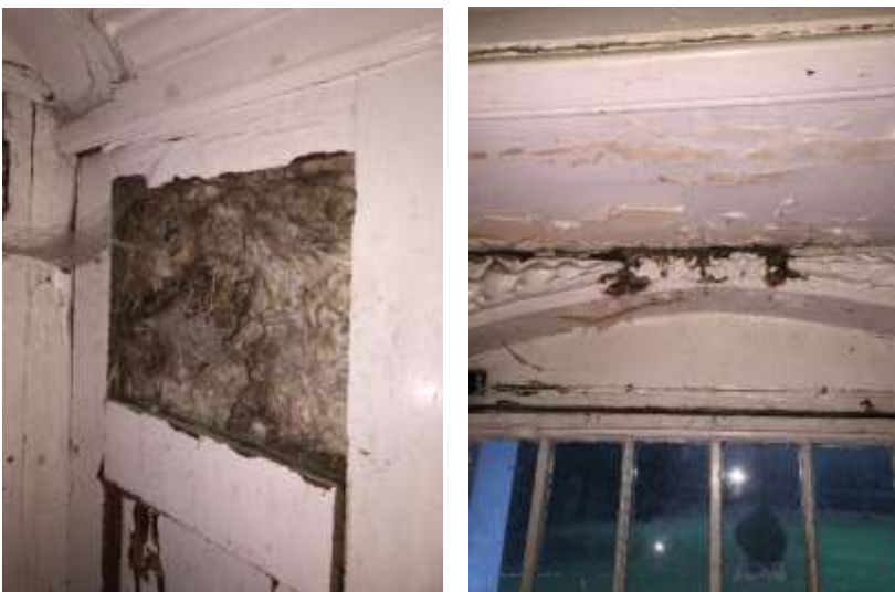
Photos 51 & 52- Entrance Hall – Rot within paneling to right of Main Entrance door surround and evident in feature paneling above door.
