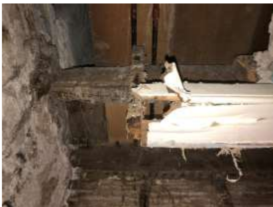
Photo 39 - Room G1 – Dry rot to left hand door frame leading to Entrance Hall.
