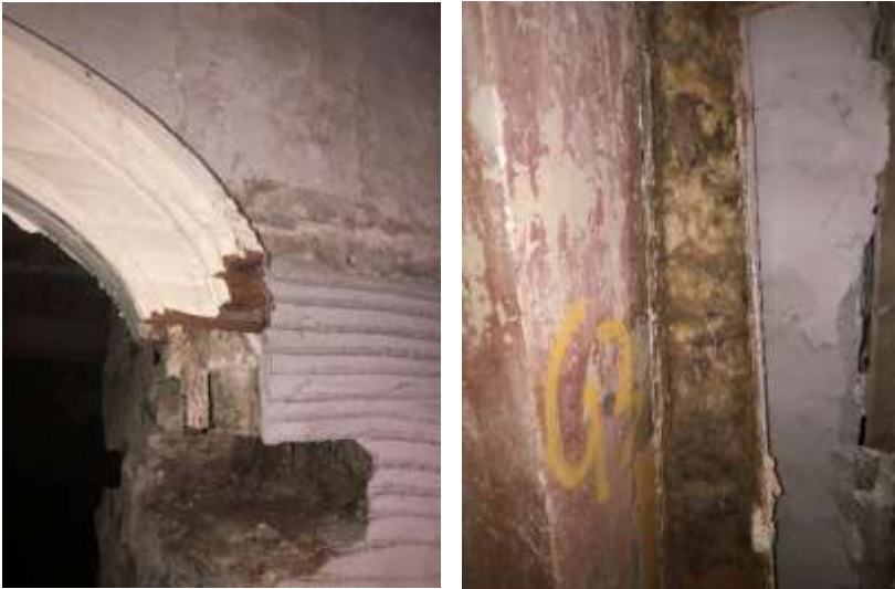
Photos 47 & 48 - Entrance Hall doorway leading to Room F5 – Rot to door surround.
