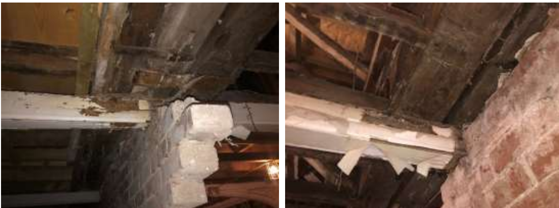
Photos 66 & 67 - Room G7 – Rot to feature arch over later addition brick wall.
