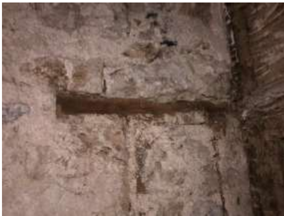
Photo 37 - Room G1 – Rotten timber lintel to previously infilled opening.
